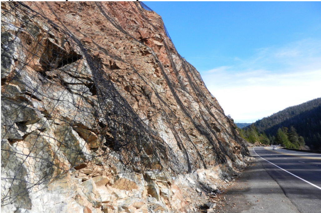
Figure 9. Example of a rock drape steel cable mesh.
