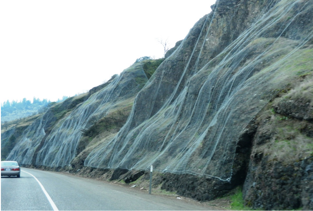
Figure 8. Example of a rock drape steel mesh.
