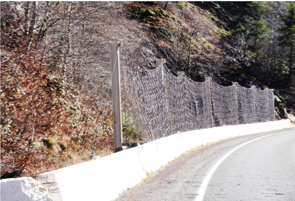
Figure 7. Example of a rockfall barrier with steel ring nets and mesh.
